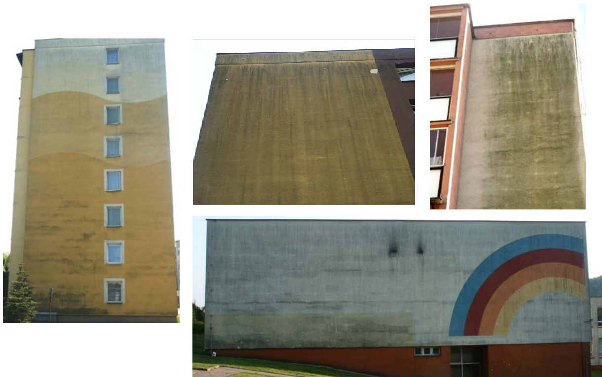
Figure 2: Algae on humid claddings of reconstructed buildings
